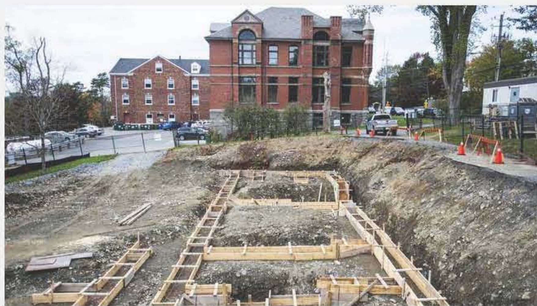
The construction site for Hospice Halifax is seen on Monday afternoon. The hospice, which is being built next to the Atlantic School of Theology in south-end Halifax, is scheduled to open in fall 2018.
